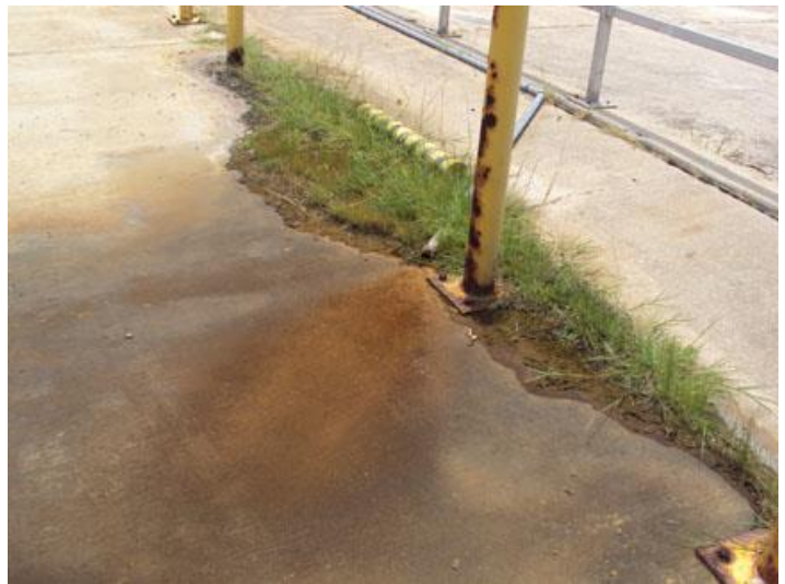
(2) Sump pump discharge point from loading dock sump.
