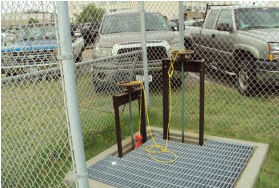
(1) Valve for wash rack
